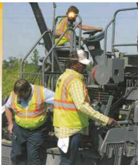
Panhandle Paving Supervisor Ernest Millender, who has 50 years of paving experience, checks the controls on the Vögele 5203-2. "This machine does things other pavers could never do," he said.
